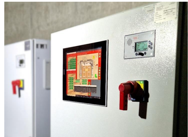
Switch cabinet with integrated touchscreen interface
